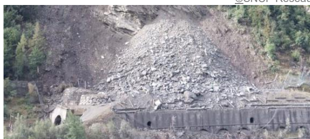
“La Brèche” railway tunnel after the landslide on 27/08/23
